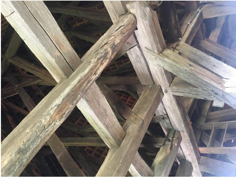
Dealu Frumos fortified Church | roof construction | the old Parts of the structure combined with the new ones.
